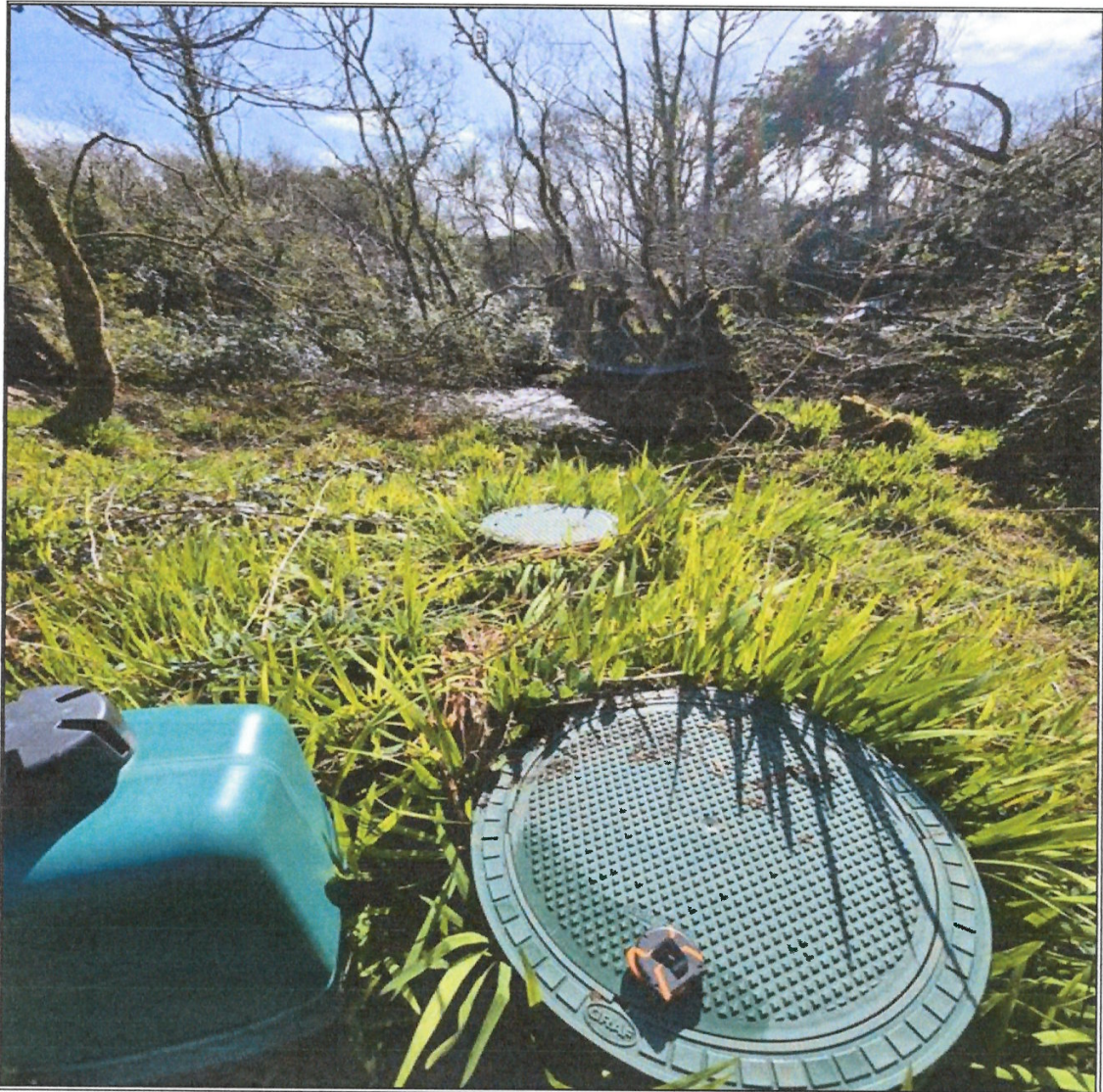
Figure 5.1: Pump measured at 8.3 meters from high water mark. The additional pump and initial filter stage at the bottom left of the picture were measured as beyond 8 meters from the high-water mark.
